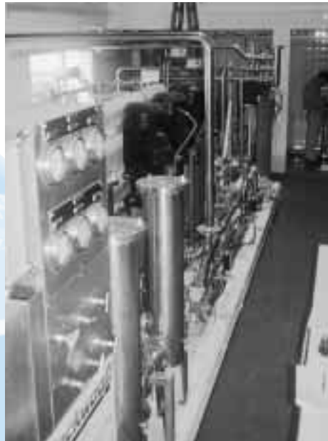
Various SIGNET measurement systems are used in the new reverse osmosis units.
